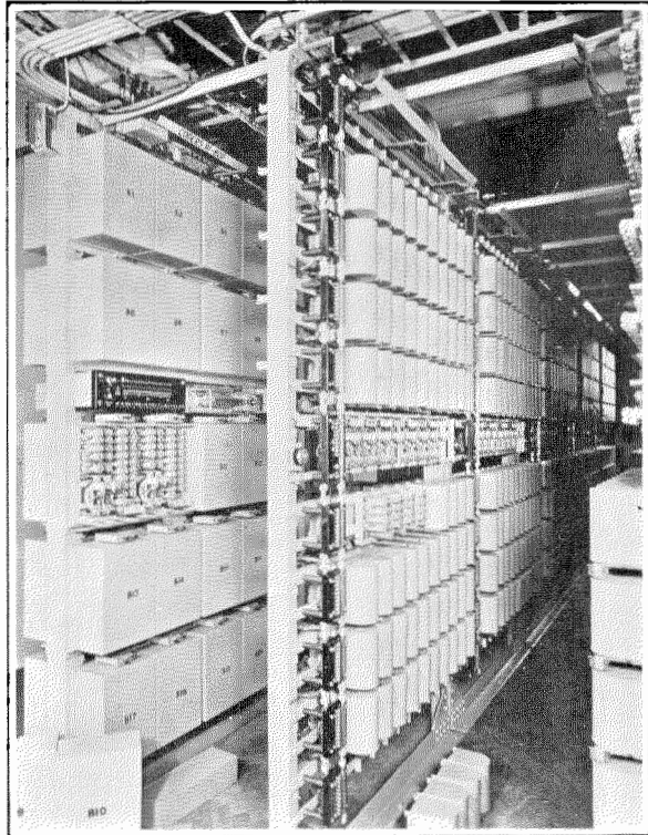
Figure 16—Coder Racks and Junction Apparatus Racks.
